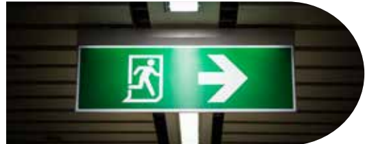
EMERGENCY AND SAFETY SYSTEMS
