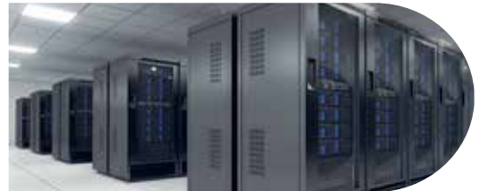
LARGE DATA CENTRE
