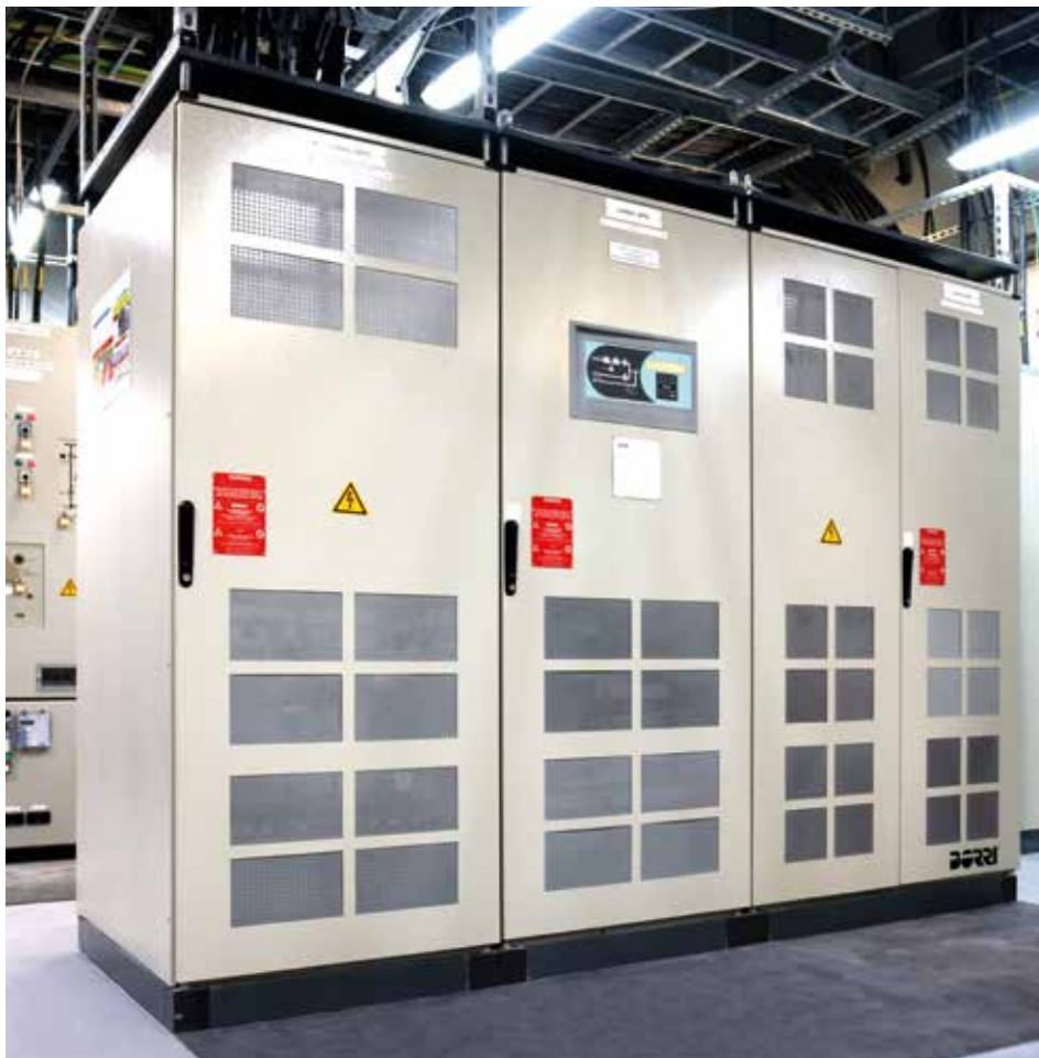
On the left: Borri AC UPS E3001.igbt 200 kW
